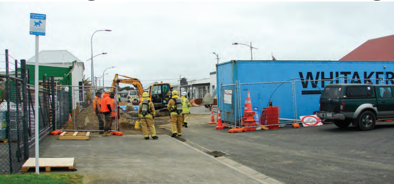
Scene of the gas leak at the Opunake Green Space project on Monday September 21.
